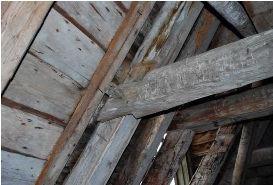
Figure 34. Connection that has lost its structural capacity. Original markings can be seen on the side of the rafter. Also, one collar beam is entirely missing from its place which can be due to obstacles in between the rafter pairs. See detail C in Figure 18.
