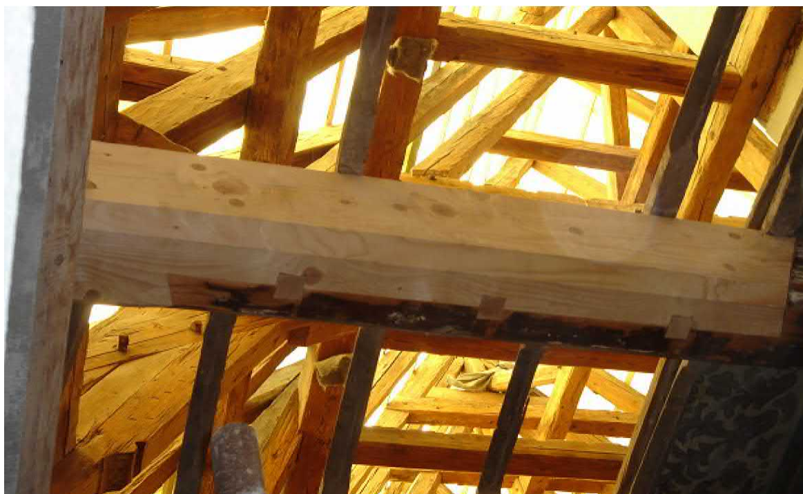
Figure 7. Removed floor joist end replaced by timber supported from masonry wall in Prague year 2007 [22, p. 69].
