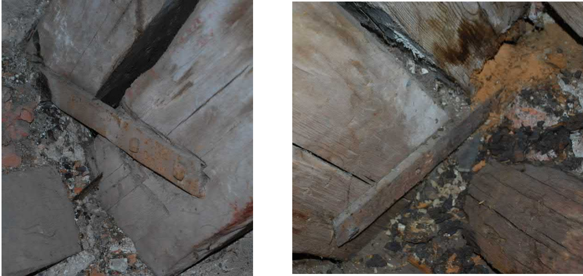
Figure 33. Rafter S86 on the left and S94 on the right are for unspecified reason connected to the posts of the leaning trestles with flat metal bar. See detail B in Figure 18.
