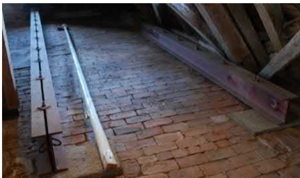
Figure 26. Two from the three steel beam pairs that were installed for additional support of tie beams in 1960.
