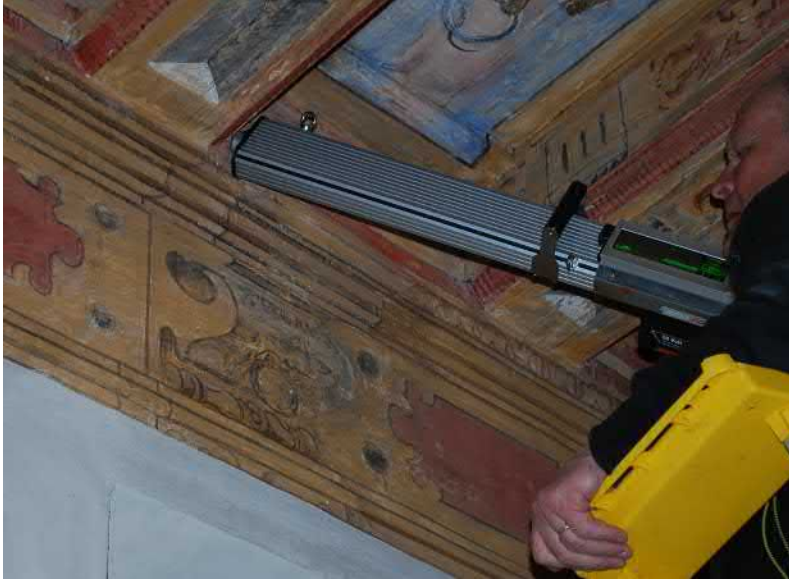
Figure 39. Resistance drillings taking place with Resistograph on the tie beam end in the third floor of Louhisääri manor.
