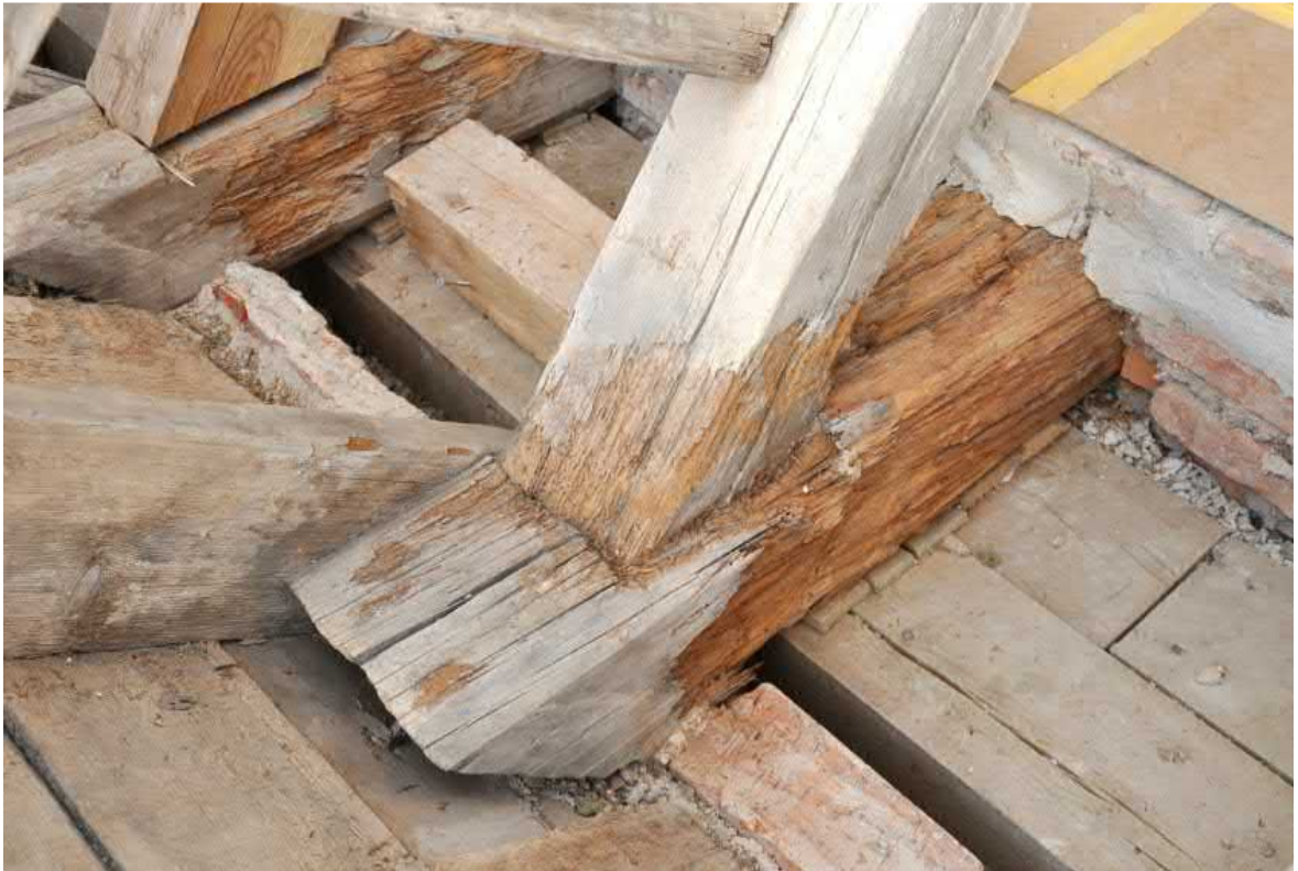
Figure 23. The rafter connecting to the tie beam in the Skokloster castle [60, p.39].
