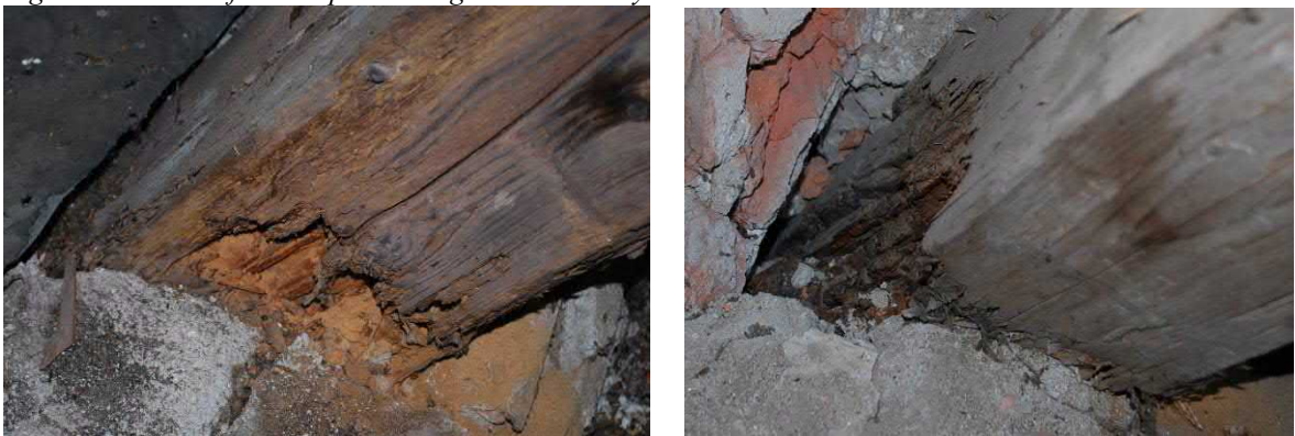
Figure 4. Left: rotten rafter S26 penetrating to the masonry wall. Right: rotten rafter S29 penetrating to the masonry wall.
