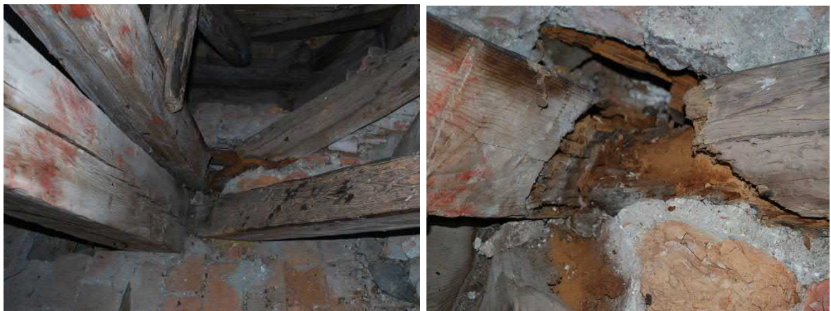
Figure 2. Left: post of the leaning trestle (VIII), rafter (S4), cross bracing and the diagonal timber member that reaches to the top of the gable. Structural opening has been made on the right side of the post. Right: showing the stage of decay more detailed.
