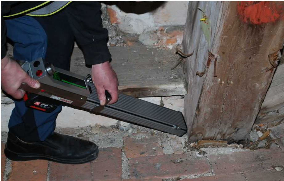
Figure 40. Resistance drilling performed to the post of the leaning trestle (PIIII) on the southwest side of the roof. The figure also shows that birch bark has been used to protect the embedded parts of the post from moisture.
