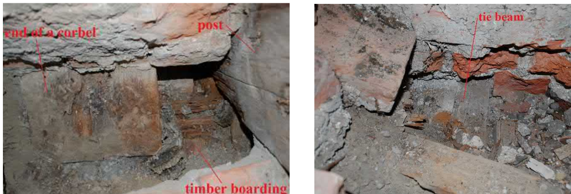
Figure 32. Structural openings that have been made in the attic. The left one is in the southeast and the right in the southwest side of the roof.
