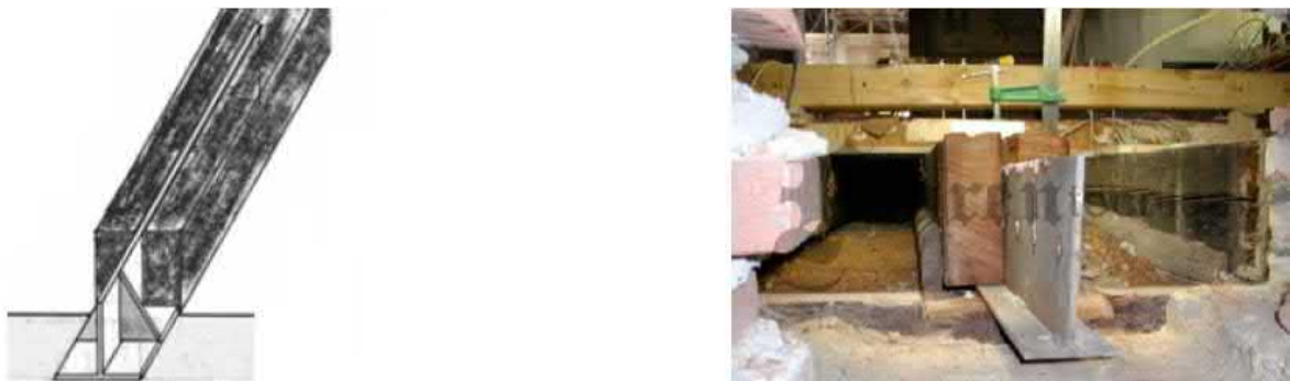
Figure 13. Deteriorated timber beam ends repaired with flitch plates [37, p. 10].
